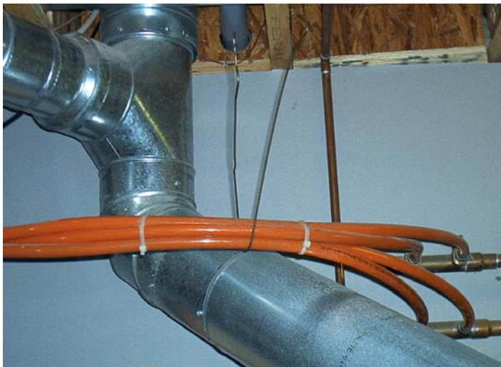
Figure 1: The galvanized pipe is venting a gas-fired cast-iron boiler.
