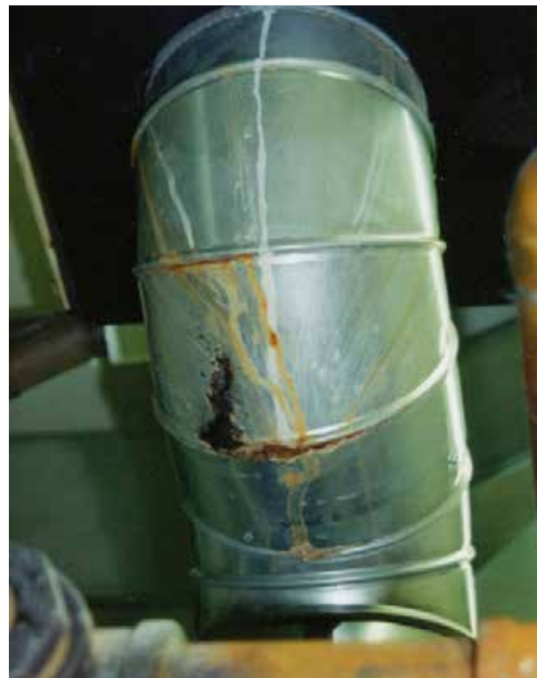
Corroded vent connector pipe after one year of operation.
